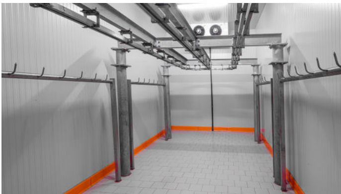
Cold Room and Storage
